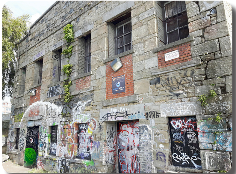
Graffiti on existing building a year ago. Demolition by neglect? Ken Johnson photo.
