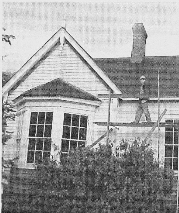
Davyd McMinn continues exterior work on Ross Bay Villa. I John Edwards photo.
