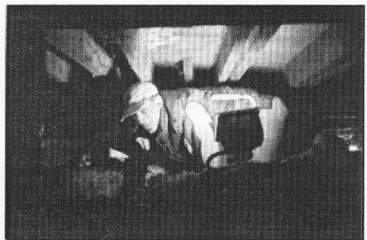
Willing volunteers work on the restoration of the foundation of Ross Bay Villa. All photos on this page by John Edwards.
