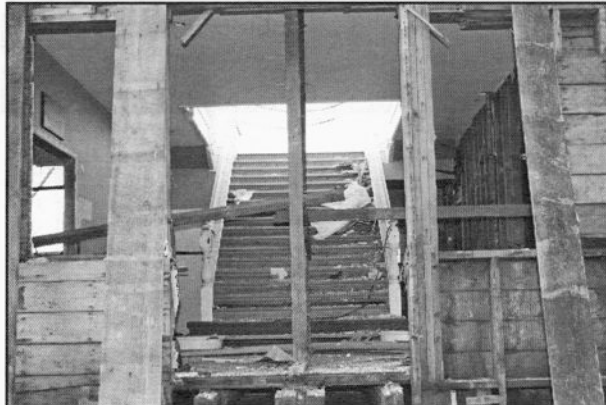
Remains of main staircase, August 20, 2006
