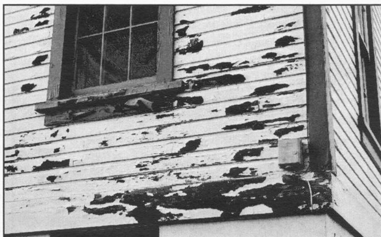
Photos: Top: Admirals's House; middle: Administration Building, 2003; bottom: detail of Administration Building, 2007 showing lack of maintenance.
