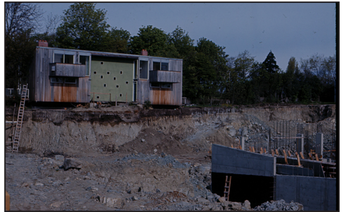
This lunar landscape represents excavations around 1980 for a James Bay highrise. But where? Donation.
