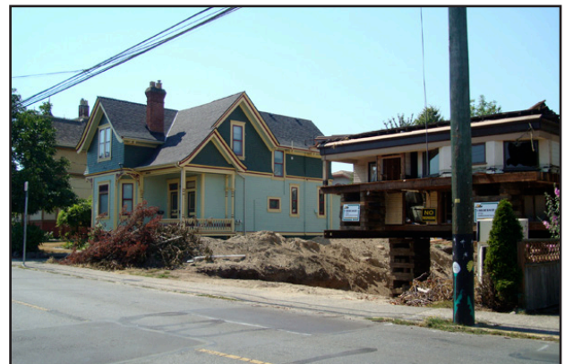
Helen Edwards photos: Left: house with upper gable folded back; right: house in process of being moved, house in new location.
