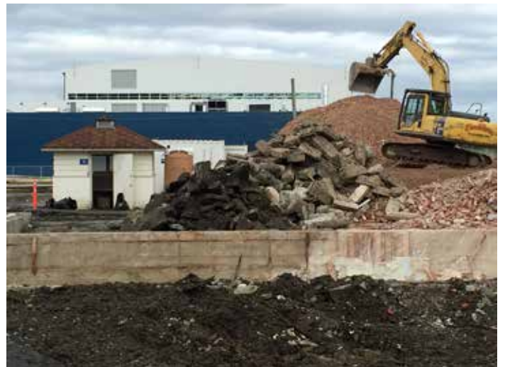
All that's left is debris
